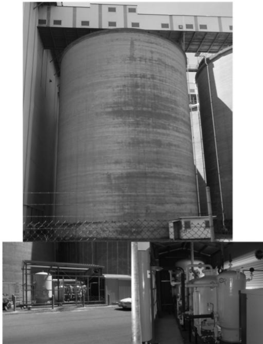
Fig. 3- A 350 m 3 /hour PSA nitrogen generator has been installed at the CBH Albany grain export terminal (35°1'50.90"S 117°53'10.54"E). The generator is plumbed to a bank of 10 × 10,000 tonne concrete cells.
